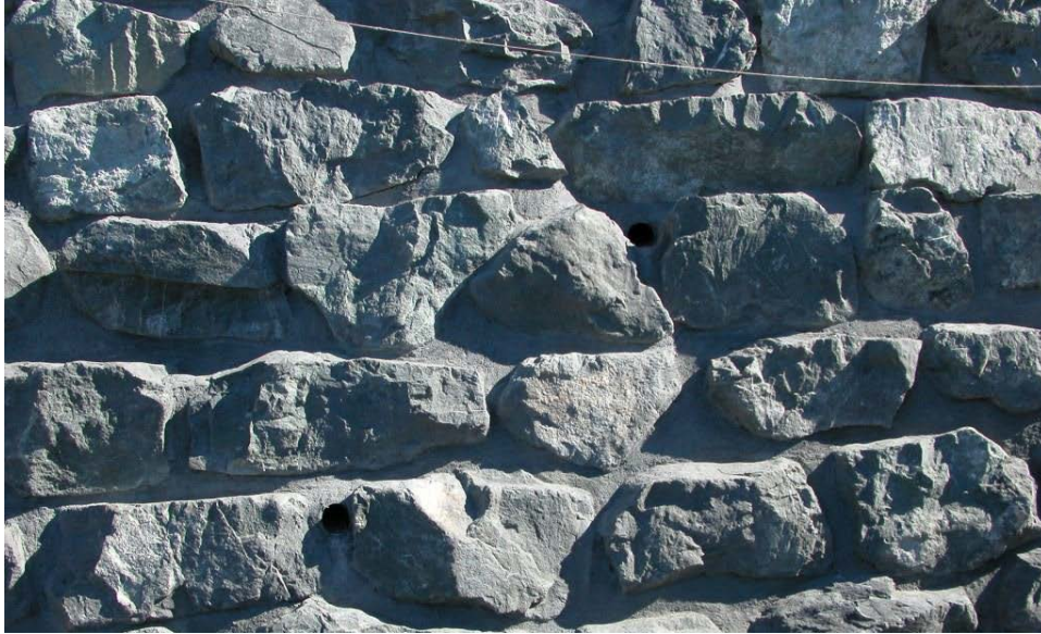
Photo 13.14 - Wet Masonry Wall
